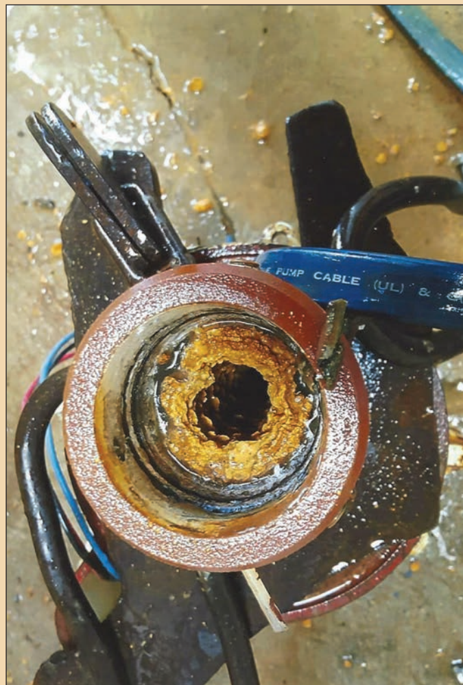
Iron oxide encrustation significantly reducing the inner diameter of a column pipe. Photos courtesy Water Systems Engineering Inc.
